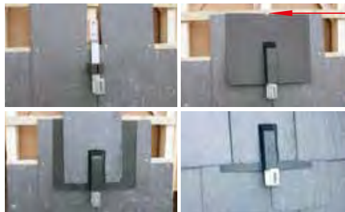
Step 4: Cut slates around the hood of the SolarFlash as per Page 4.
