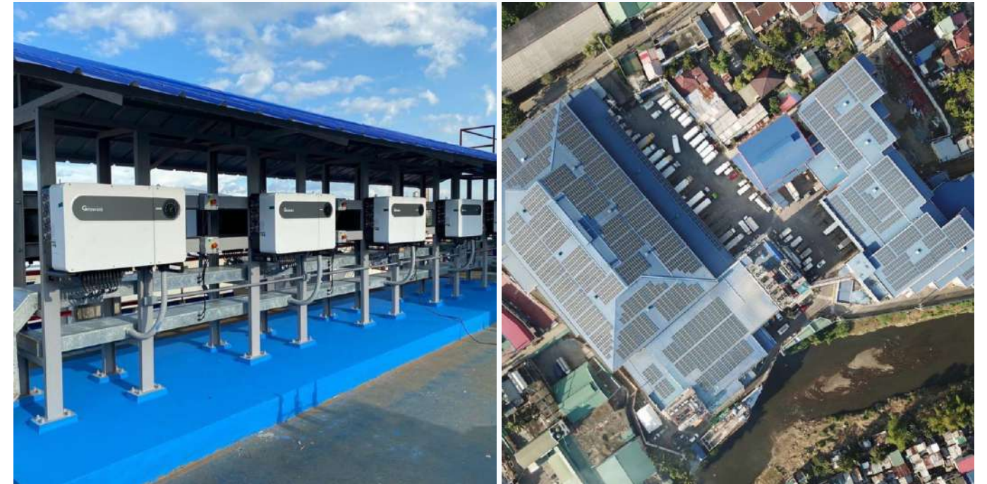
CASE STUDY: Philippines with 1.2MW solar installation.
