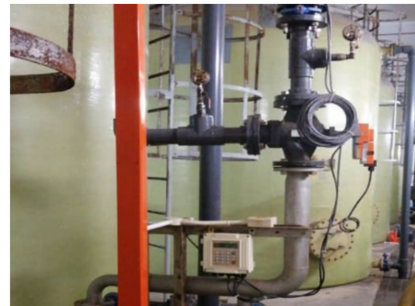
Figure: RO rejected water system
