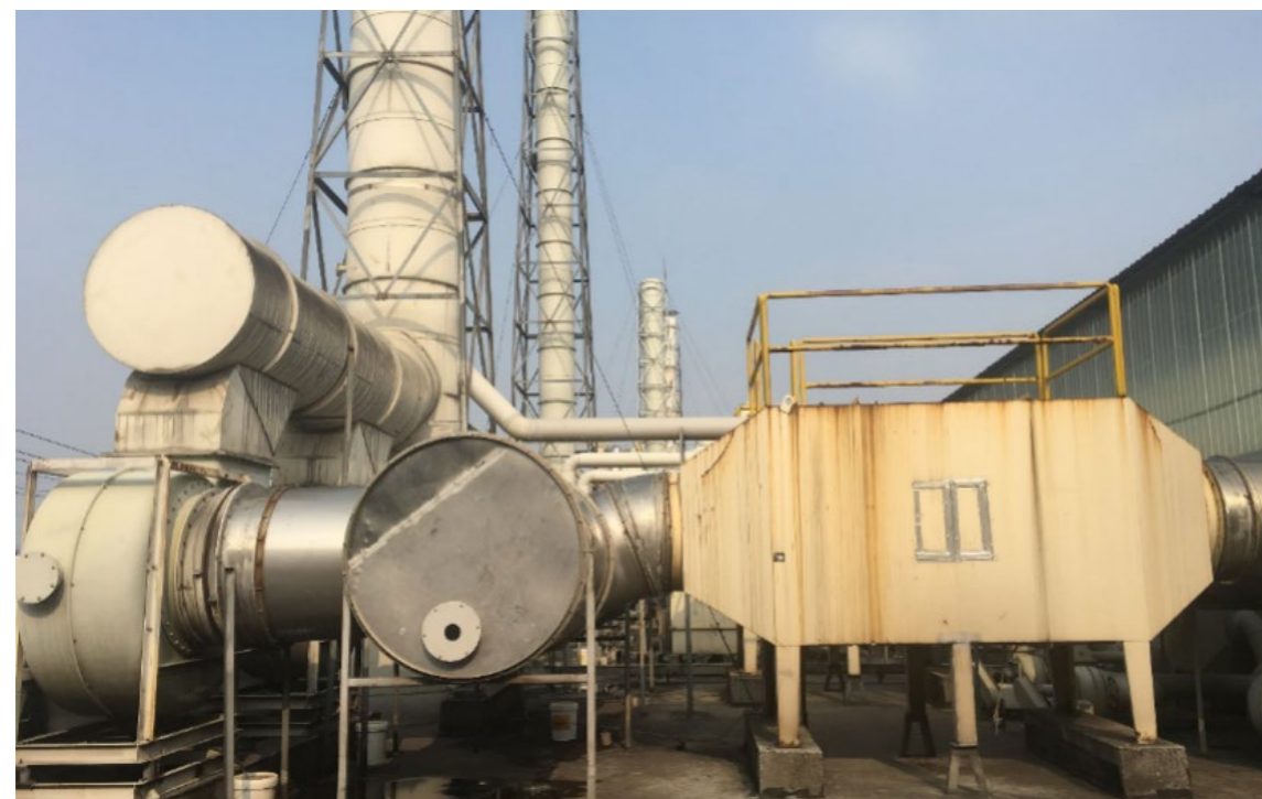
Figure: VOCs treatment system of Haining base
