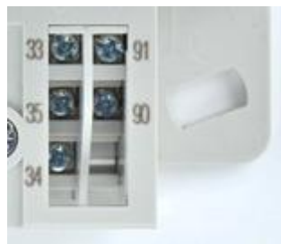
Figure 60: Service control terminal
