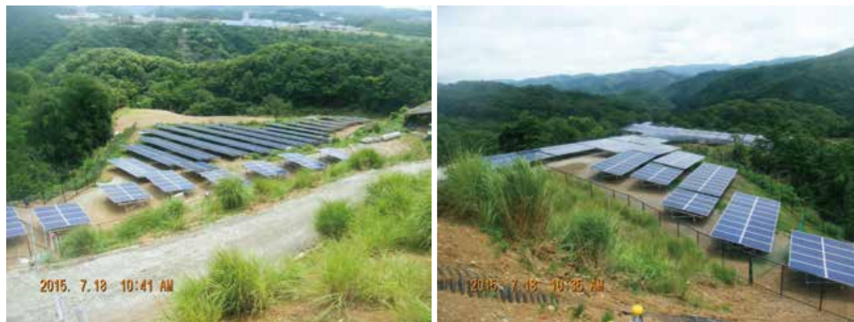
East-West Slope, AG4 + Ground Screw, 1.16MW
