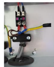
Screens crimped together but not earthed at all other points
