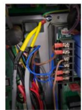
Screen Earthed in Outdoor unit
