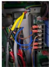
Screen Earthed in Outdoor unit
