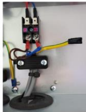
Screens crimped together but not earthed at all other points
