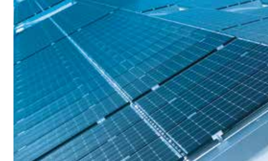
1. Photovoltaic modules on the roof generate sustainable energy for production facilities and office buildings.
